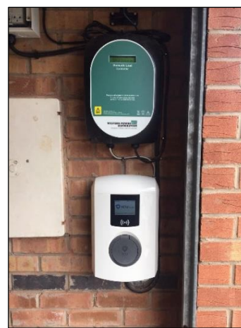
Figure 3: Example installation of controllable EV fast charger (0 – 32A single phase) and Domestic Load Controller devices in a customer's home
