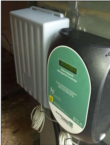
Figure 4: Example LV substation monitor
